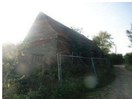
Picture 1.10 Copse Farm Barn is in need of restoration
